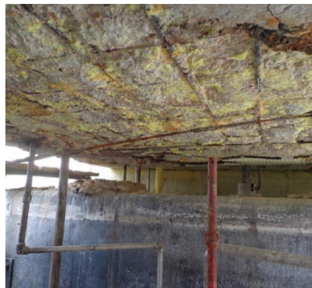
Concrete roof soffit showing severe steel reinforcement corrosion and concrete spalling. Sulfur is also infiltrated within the concrete.
